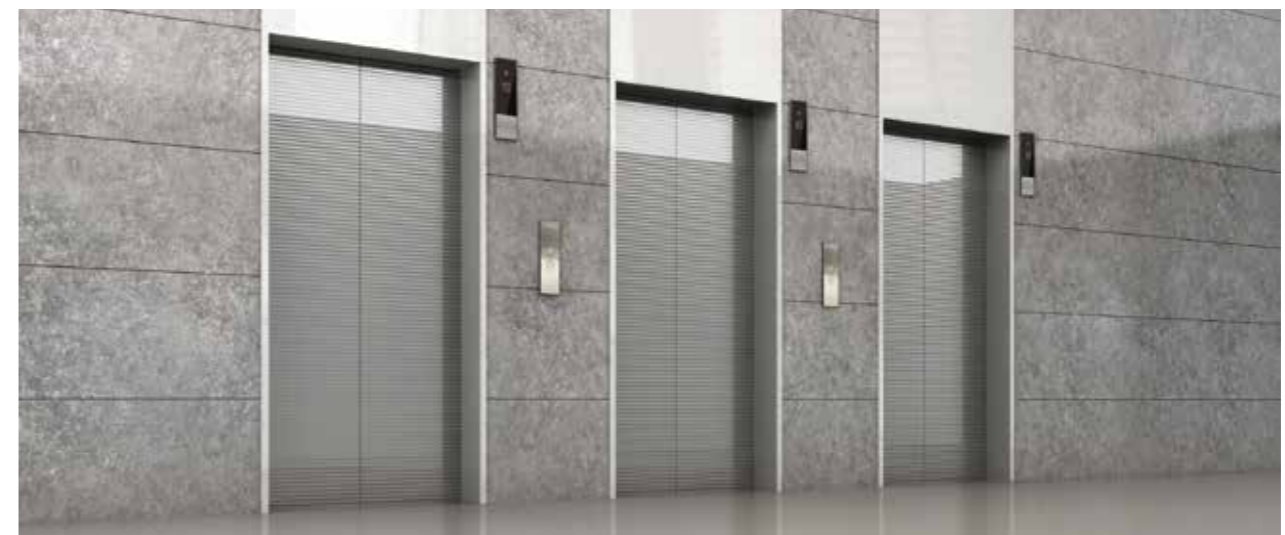
Group Supervisory Control
